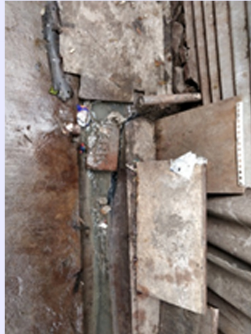
Gutter opposite their house
